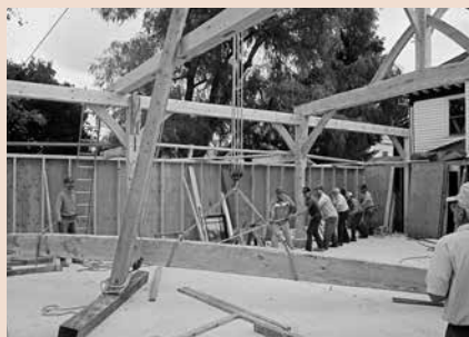
One of the big tie beams is being raised by six lodge brethren. The six-part block and tackle multiplies their force by six times. Note the pulley at the base of the gin pole that changes the direction of pull to horizontal.
