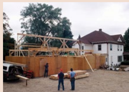
At the end of the day, the walls are buttoned up by the general contractors (Emerson Brothers). The 50' ridge beam will be supported at its ends by the gable stud walls. Note the gin pole on the truck roof at left.
