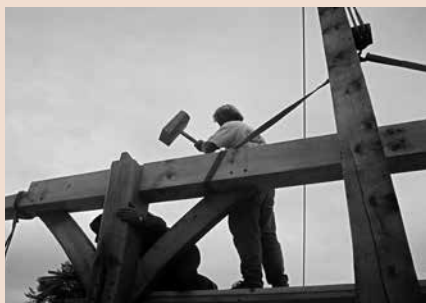
Here a section of the purlin plate has been set on the post tenons and is being "persuaded" home by Dave Bowman wielding a large wooden mallet called a persuader, beetle, or commander.
